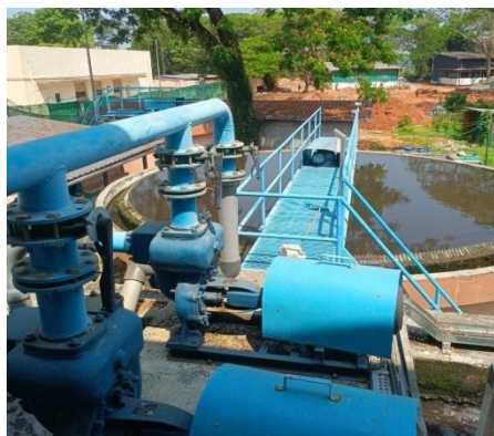
500 KLD STP at Kozhikode medical College
