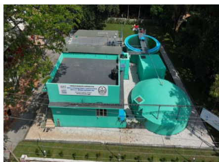
360 KLD STP at General Hospital, Thrissur
