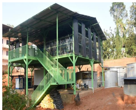
1 MLD STP at Kozhikode medical College
