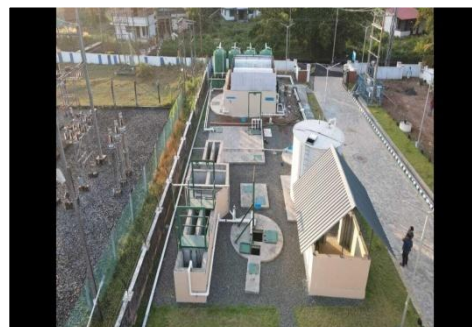
1 MLD CSTP at Padanappalam, Kannur
